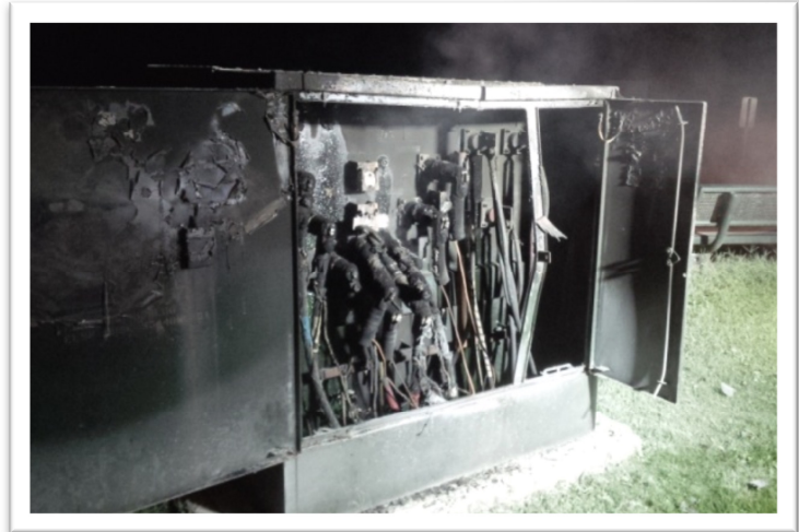
FIGURE 6.20 – 2013 TRANSFORMER FAILURE ON JEANNE D’ARC BOULEVARD
