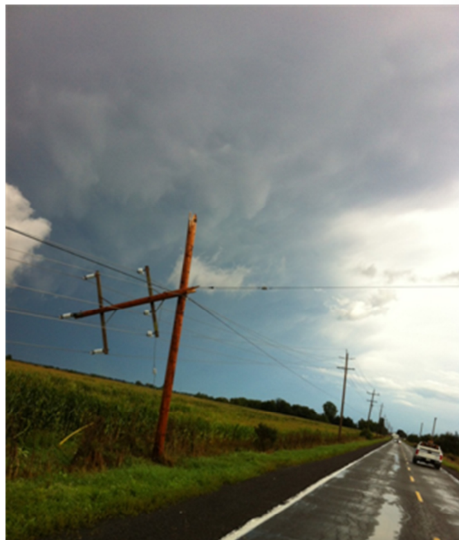
FIGURE 6.4 - 2013 POLE FAILURE ON SHEA ROAD
