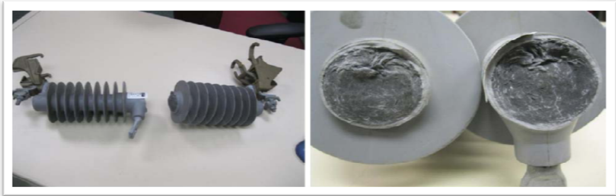
FIGURE 6.34 - FAILED S& C SMD-20 SWITCH
