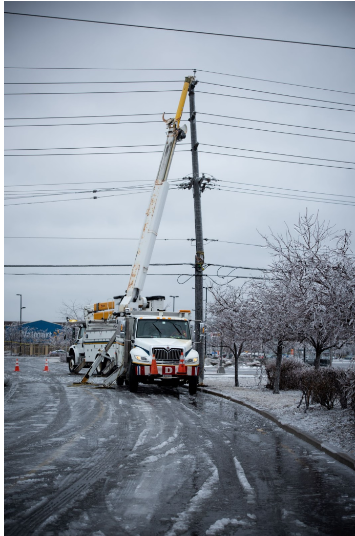
Figure 2.9 – Pole Replacement Following 2018 Ice Storm
