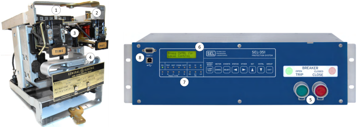
Figure 6.17 – Station Protective Relays
